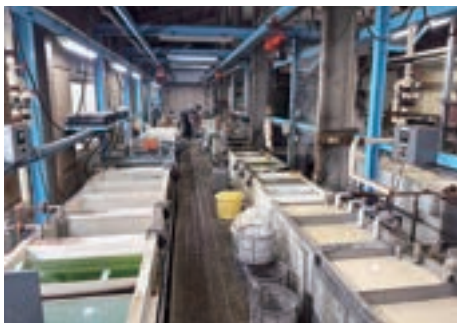
Plating lines capable of handling a wide variety of combinations
